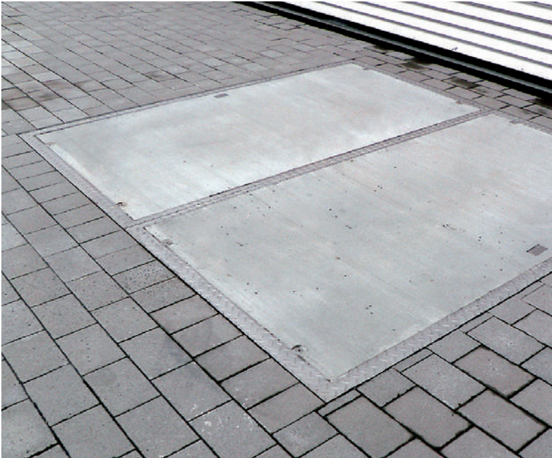
Two-piece shaft cover with concrete surface – Frankfurt
