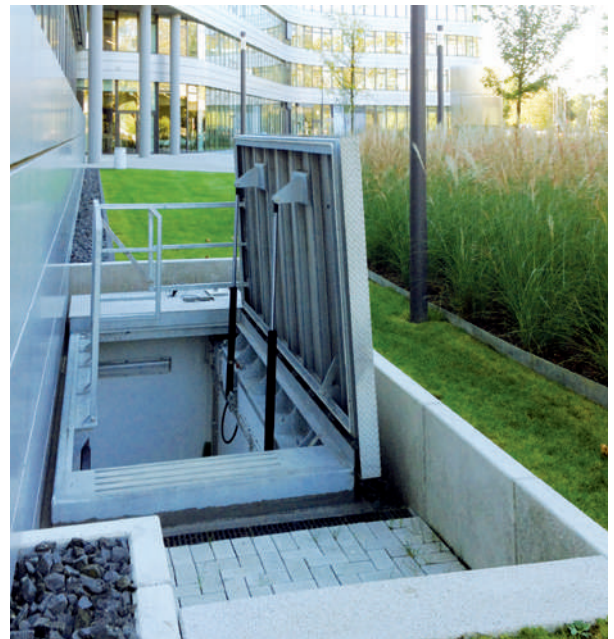
Hydraulic stainless steel escape hatch – Cologne
