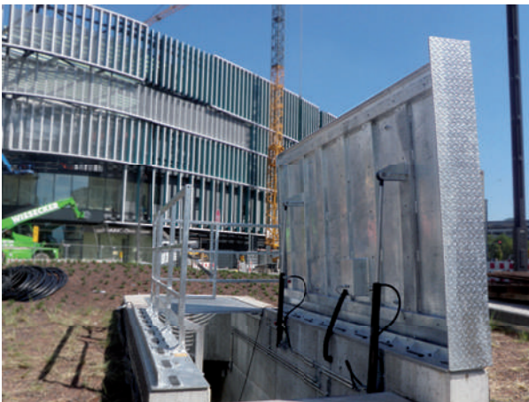
Hydraulic escape hatch – Frankfurt
